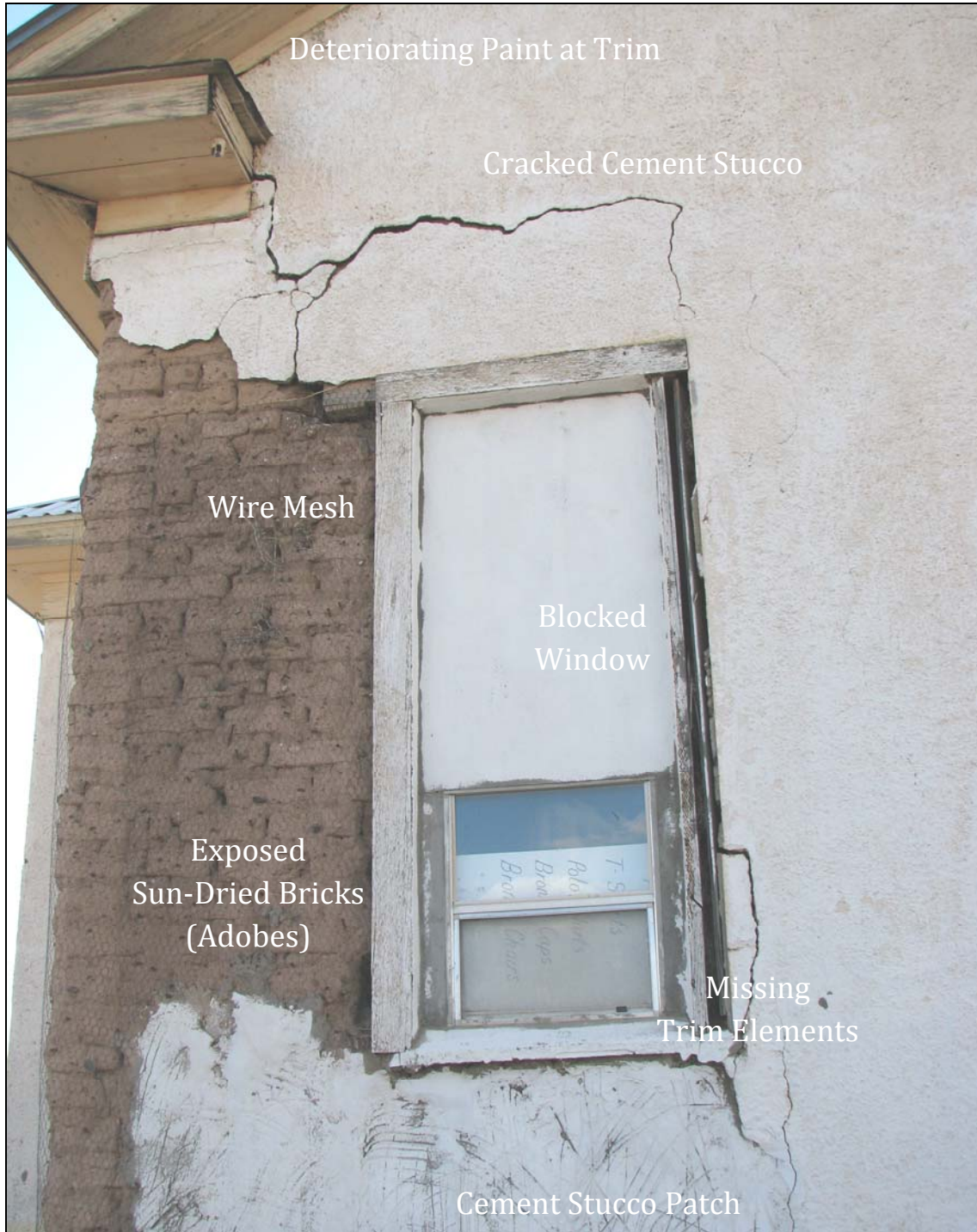
Deterioration at Front Façade Caused by the Addition of Cement Stucco
