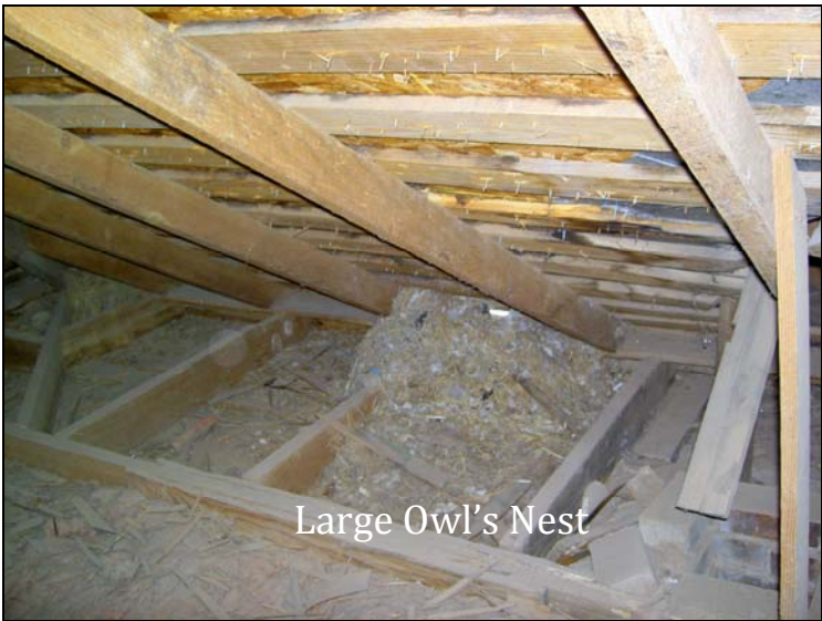
Photo (left) Shows Large Owl's Nest at Roof Eave. A Missing Piece of Rake Trim/Cornice Return at the Exterior Front Façade Has Allowed the Intrusion
